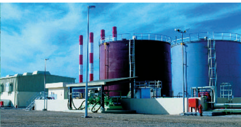
Fuel storage area
