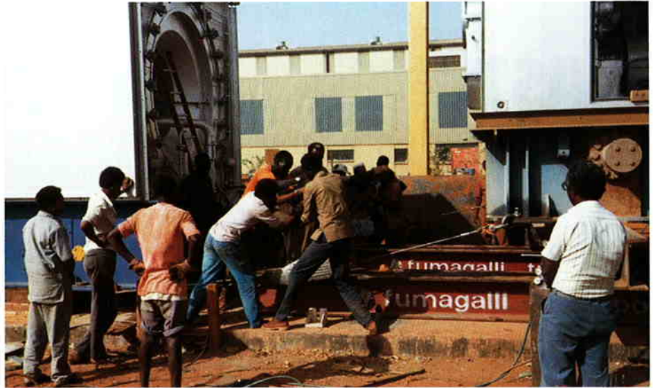
Installation and alignment of gasturbine (90 t per unit) and generator ► (103 t per unit).
