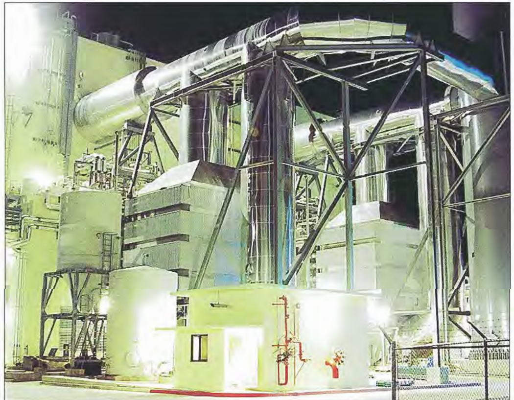
The boiler area
