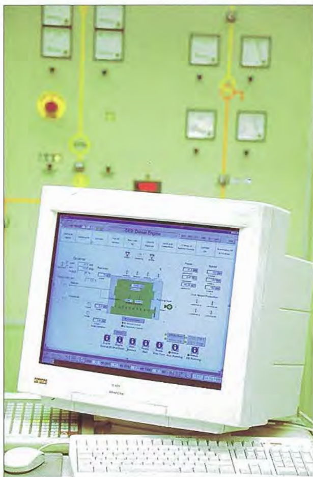
Power Generation Control – Video Display Unit (VDU)
