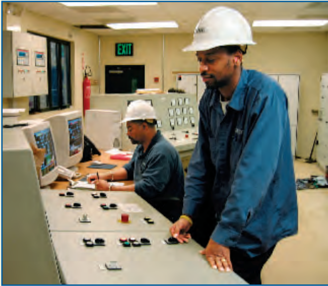
Control room operation
