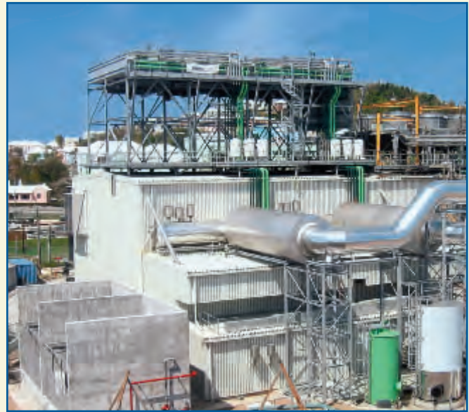
Radiator coolers on roof
