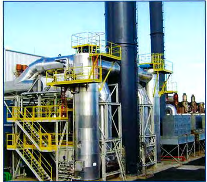
Exhaust gas boilers
