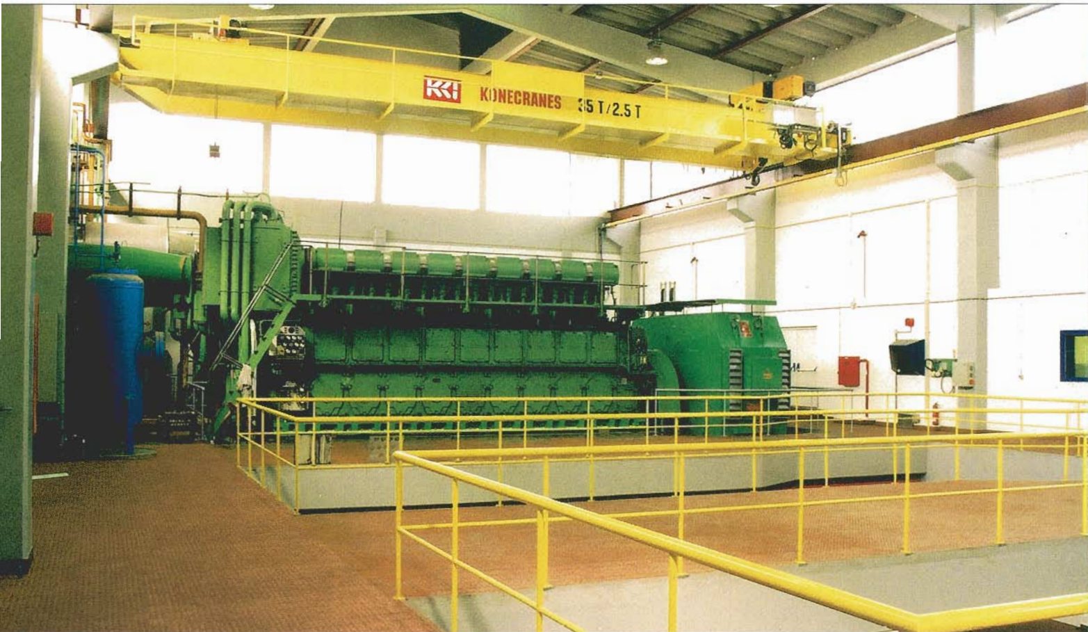
Engine Hall view of the two 9L 40/54 engines and the space for additional two engine foundations.
