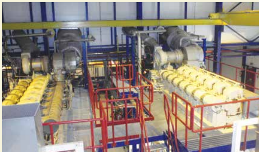
Engine hall with Unit 7 to the right.
