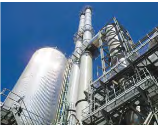
Abatement and stack area.
