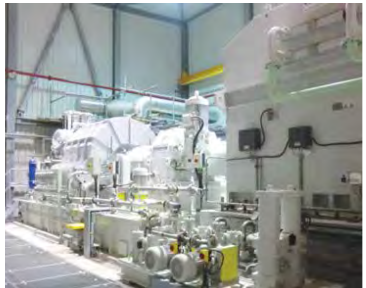
Steam turbine generator.
