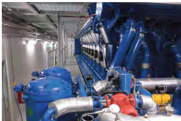
Engine in noise enclosure.
