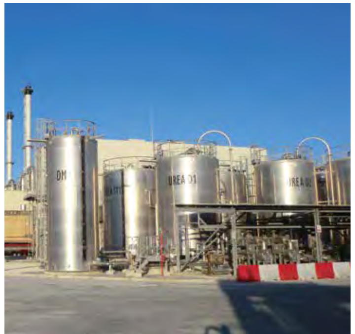
Urea solution preparation tanks.
