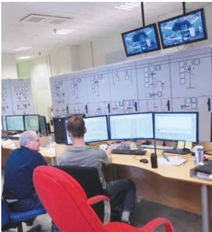
Plant control room.
