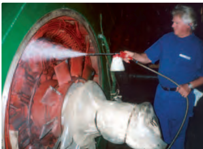
Khashm El Girba Power Station in the Sudan. Major overhaul of generator.
