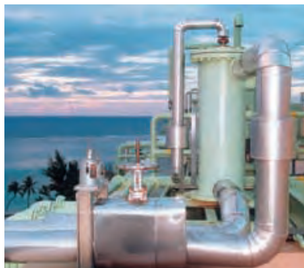
Fuel oil venting tank.
