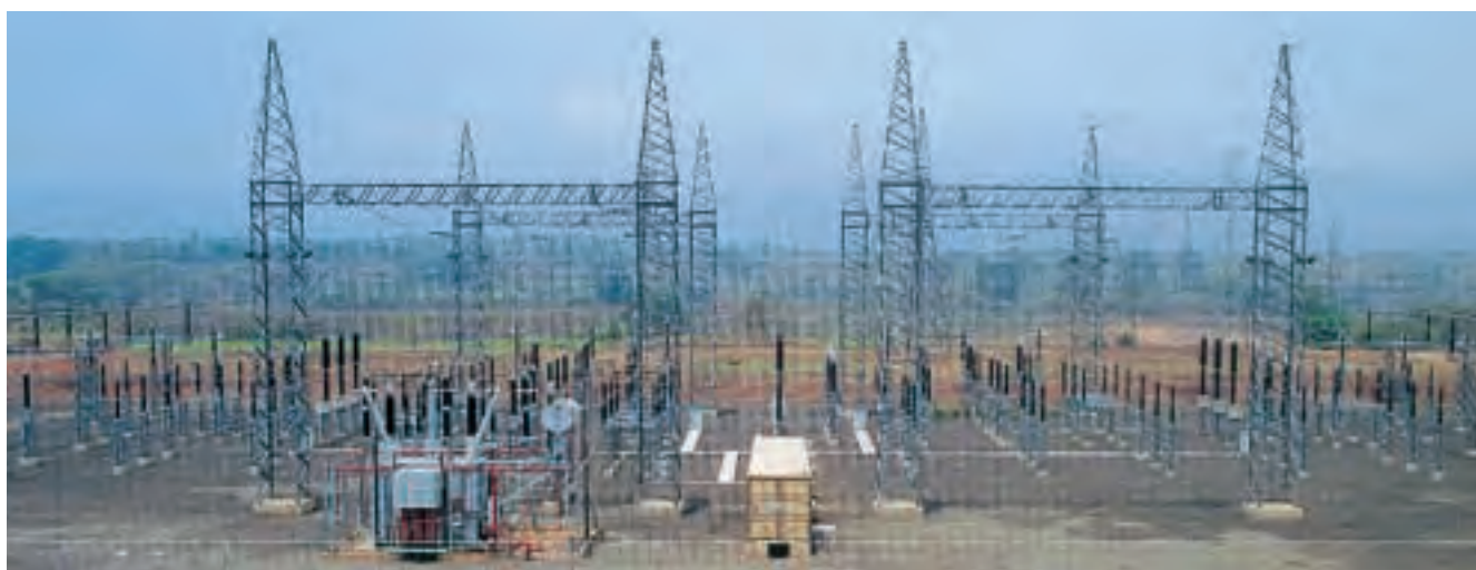
Transformer Station - Pacora Power Station, Panama.
