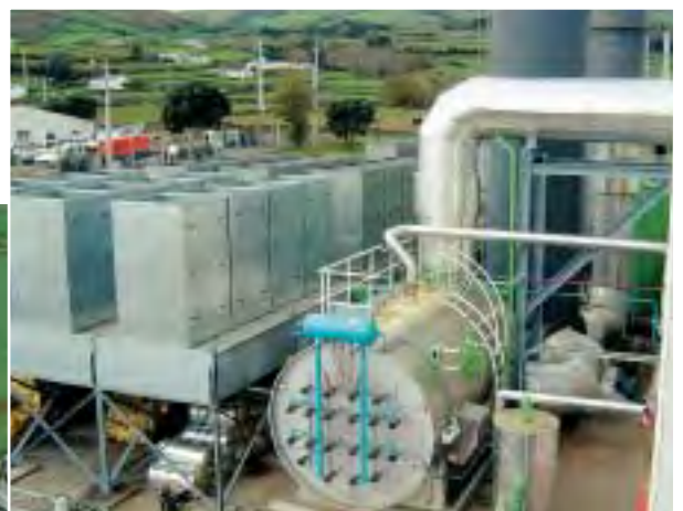
Belo Jardim New Boiler Plant, Unit 5, Terceira, the Azores.
