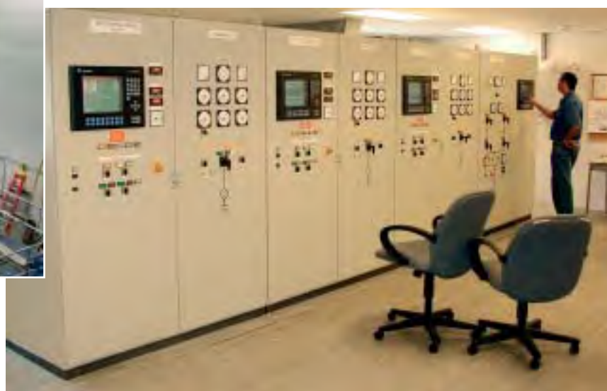
Control room, Grand Cayman.
