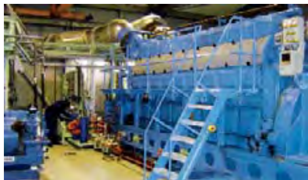
Engine Hall, Pointe Monnier Power Station, Rodrigues, Mauritius.
