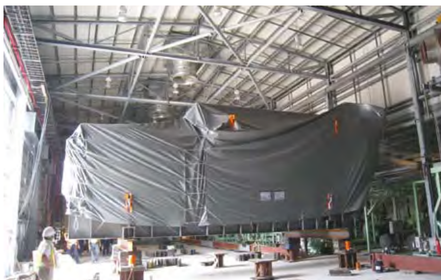
West Sunrise Power Station, Grand Bahama
